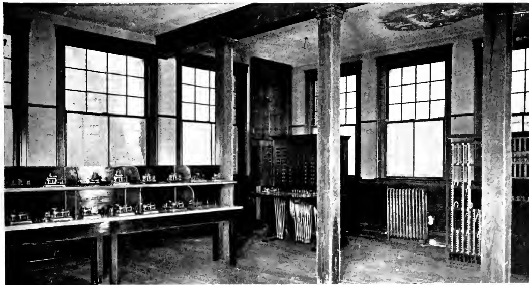
FIG. 20.—VIEW OF WIRE CHIEF'S ROOM, THOMPSON'S CORNERS, O., SHOWING REPEATER TABLES, TEST PANEL AND PORTION OF COIL RACK.
